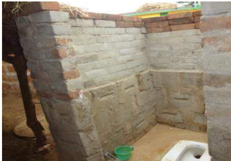
A Toilet without a Door and Roof
